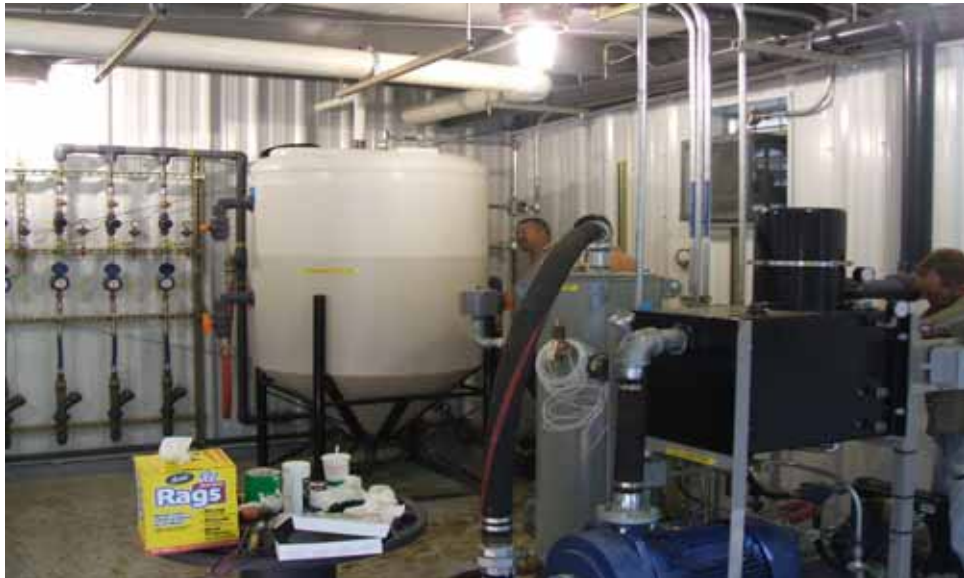
View of liquid ring pump, moisture separator and settling tank
