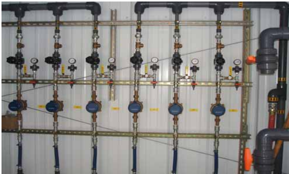
View of building interior and of SRW and DRW series well manifolds
