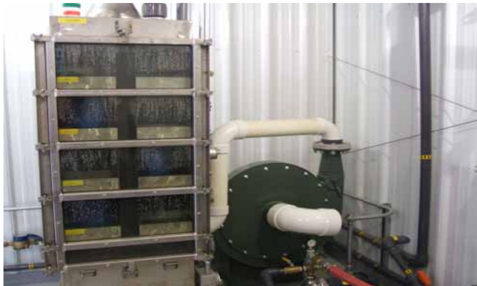
View of air stripper unit
