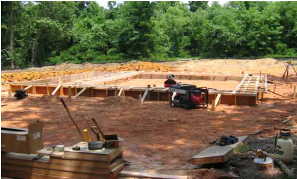
View of forms for concrete pad. Left side of pad is future equipment control room. Right side of pad will contain groundwater treatment equipment
