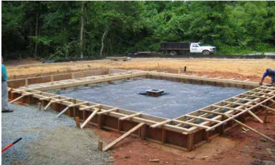
View of forms for concrete pad. Moisture barrier is present and underlain by crushed rock
