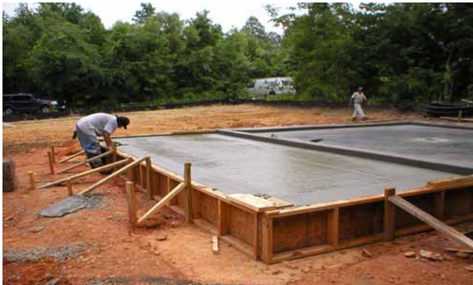
View of slab. Equipment control room in foreground and equipment room in background
