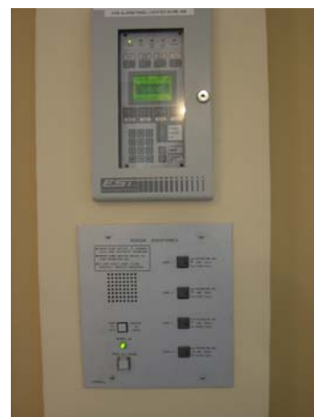
Graham Memorial Hall Fire Alarm Panel (upper) works in conjunction with the Area of Rescue Assistance Control Panel (lower).
