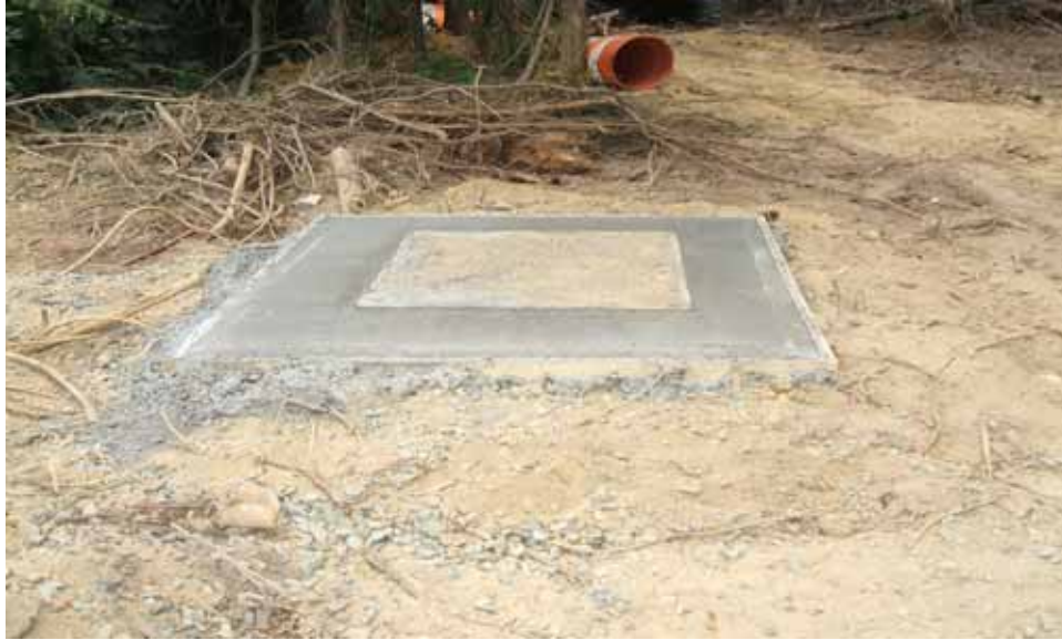
View of vault and pad on VER well
