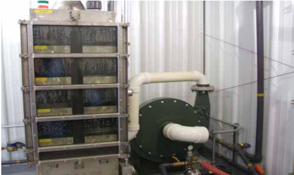
View of air stripper unit
