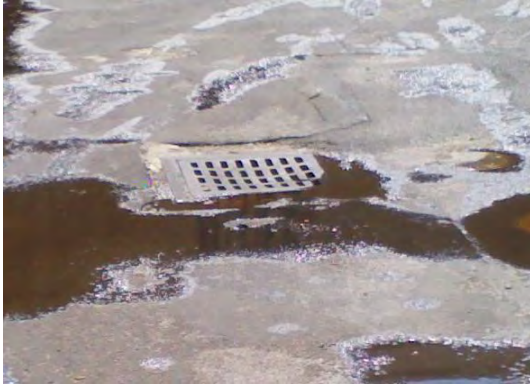
Kitchen grease spilling into a storm drain on campus (2012)
