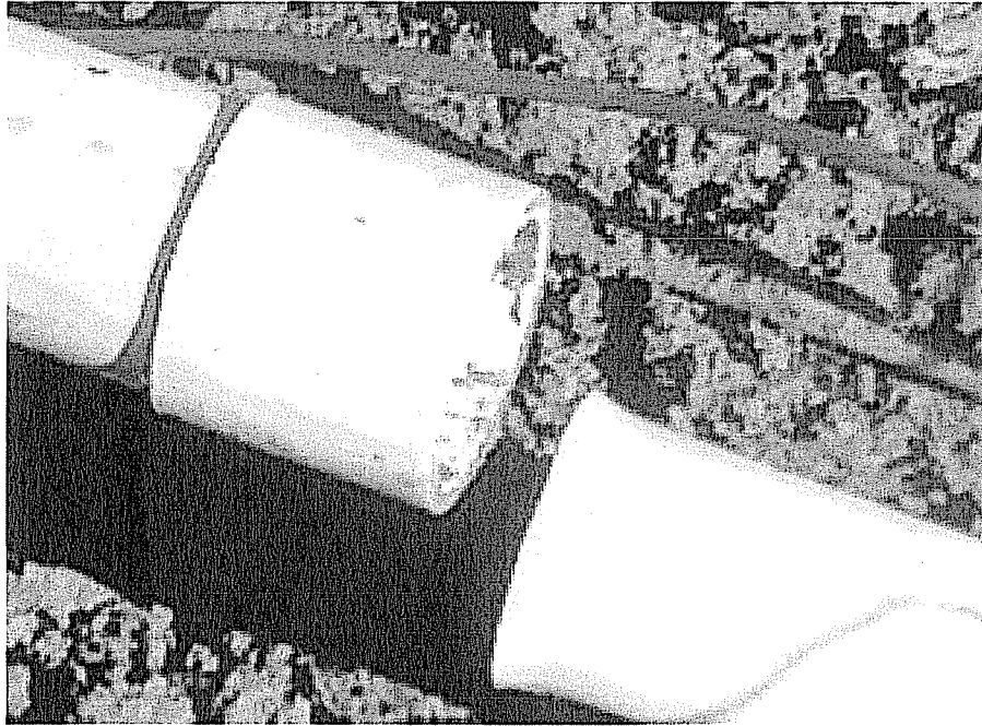
Picture 1 – Broken bell fitting.
