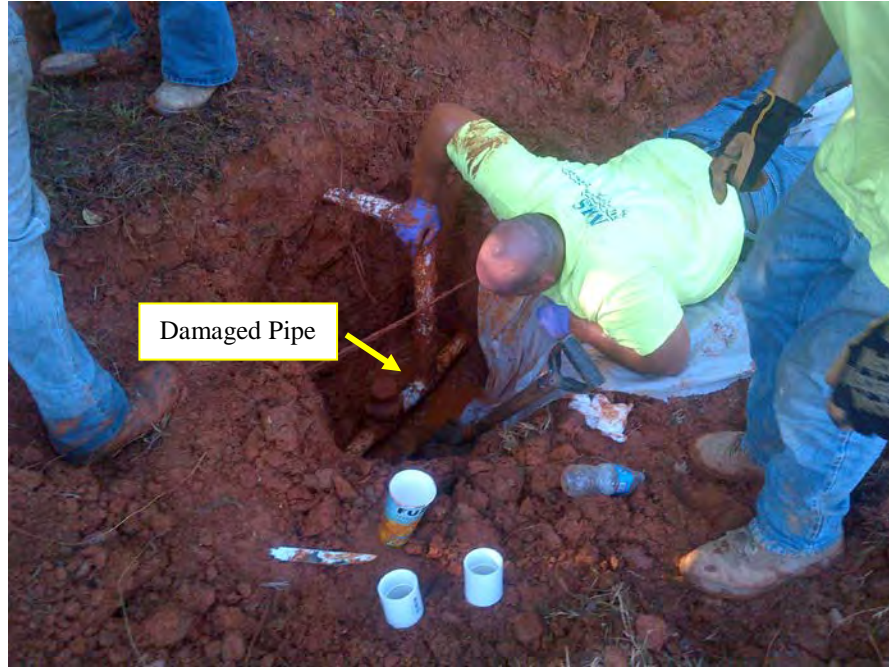
Picture 1 – Damaged 2-inch force main.
