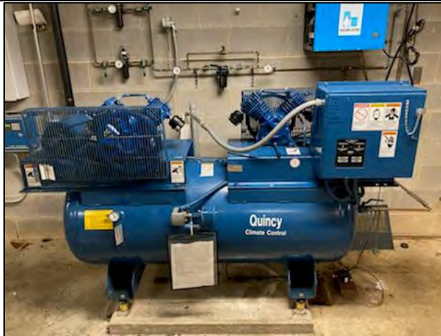
Example: Koury Residence Hall, Basement Mechanical Room
