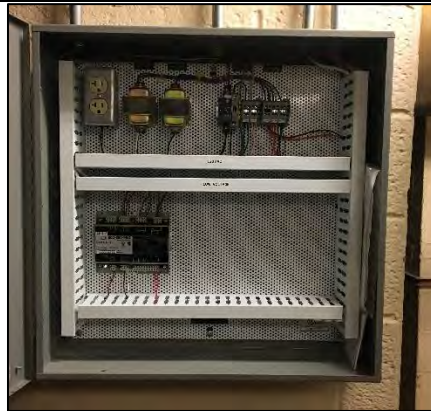
Example: Rosenau Hall, Air Handler #6
