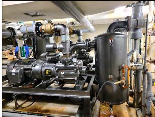
Example: Brauer Hall Vacuum Pump and Separator Tank
