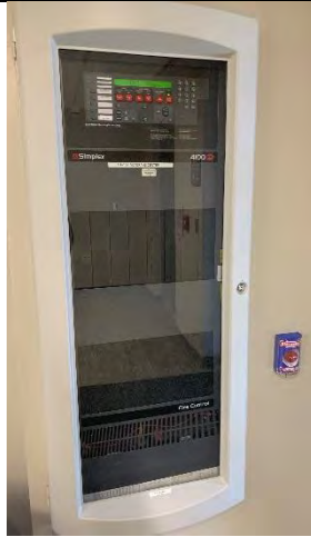
Fire Alarm Control Panel
