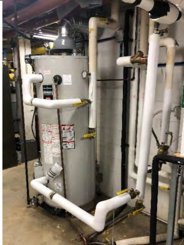
Example Location: Glaxo Building, Mechanical Room
